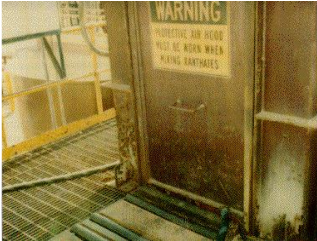
Door and rollers used for the emptying of drums into the mixing tank.
