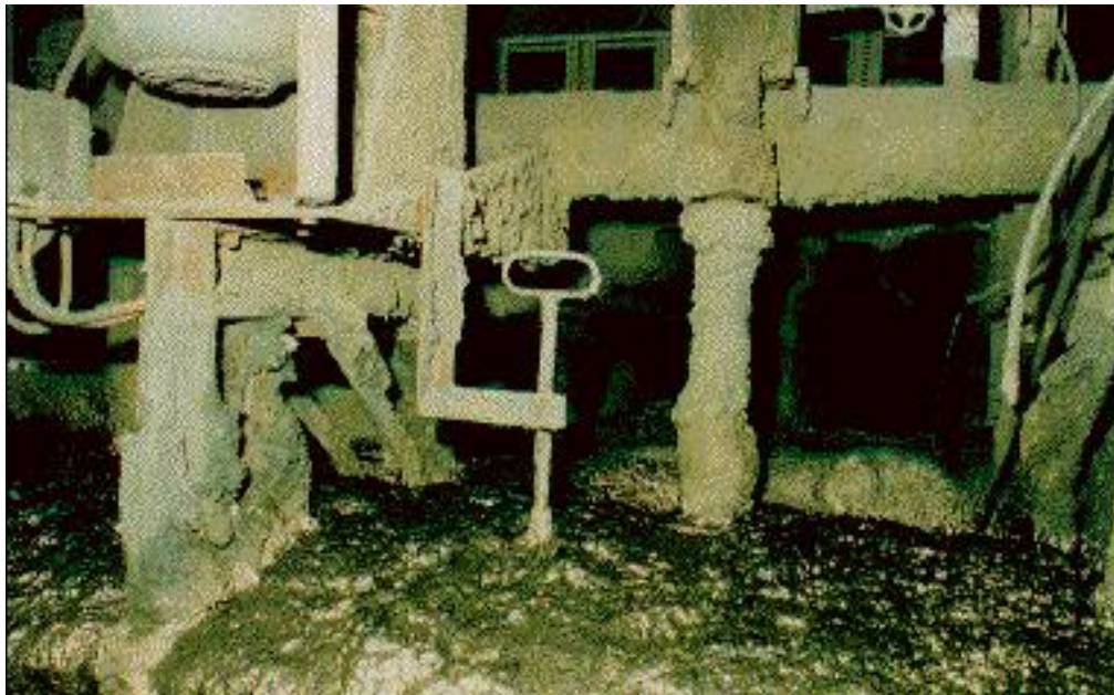
Flotation cell showing sodium ethyl xanthate addition point at right of centre.
